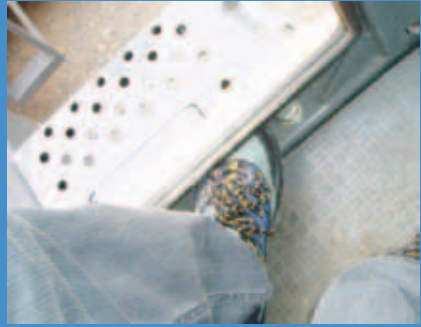
4. This cabin has a tripping hazard on exit.
